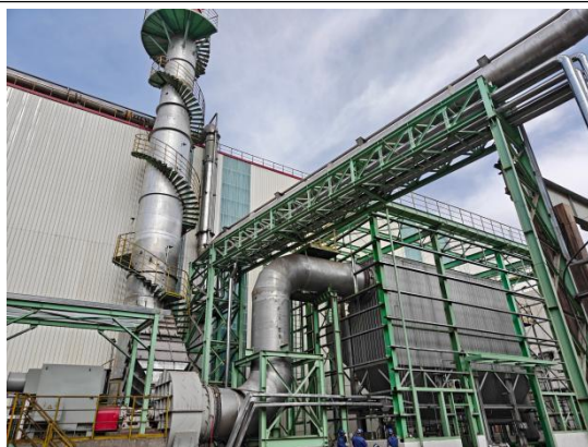
粗轧机除尘+排气筒
